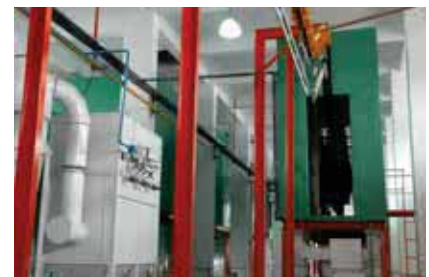
Sheet Metal Pre treatment Facility for Canopy to prevent rusting.
